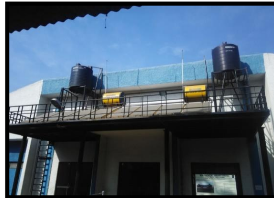
4. SOLAR WATER HEATER IN CANTEEN.
