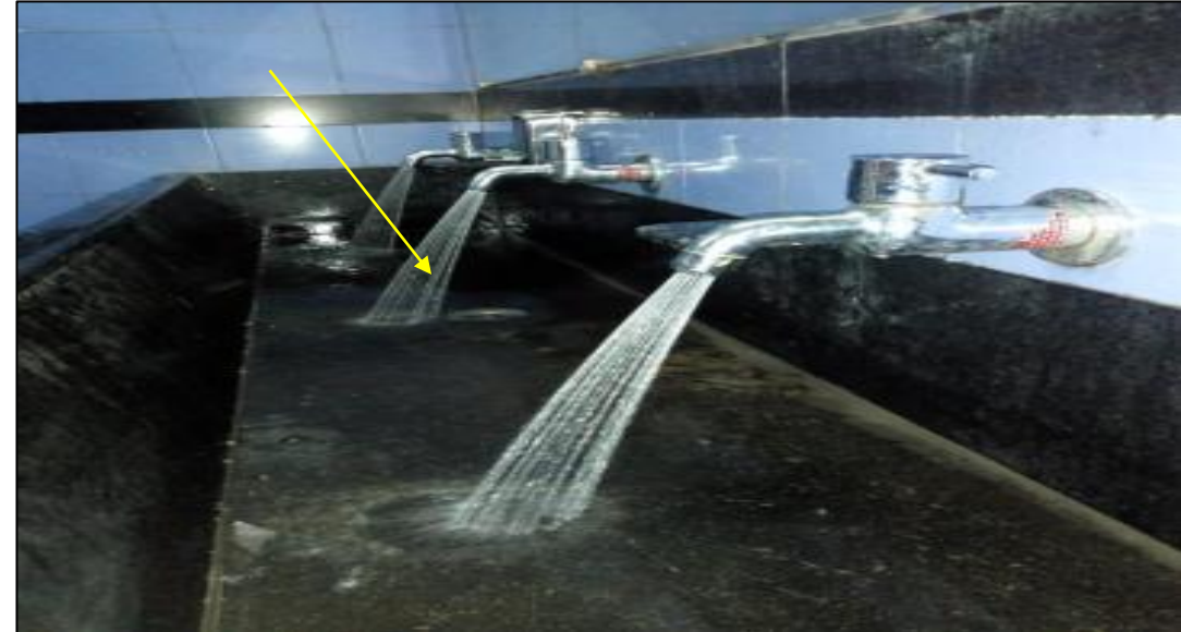
Installation of water saving sprinkler nozzle for water taps - Saving 300 ml water per use
