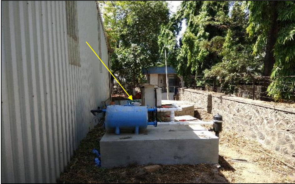
Reuse of ETP processed water for gardening with the help of drip irrigation @ 5-6 KL per day
